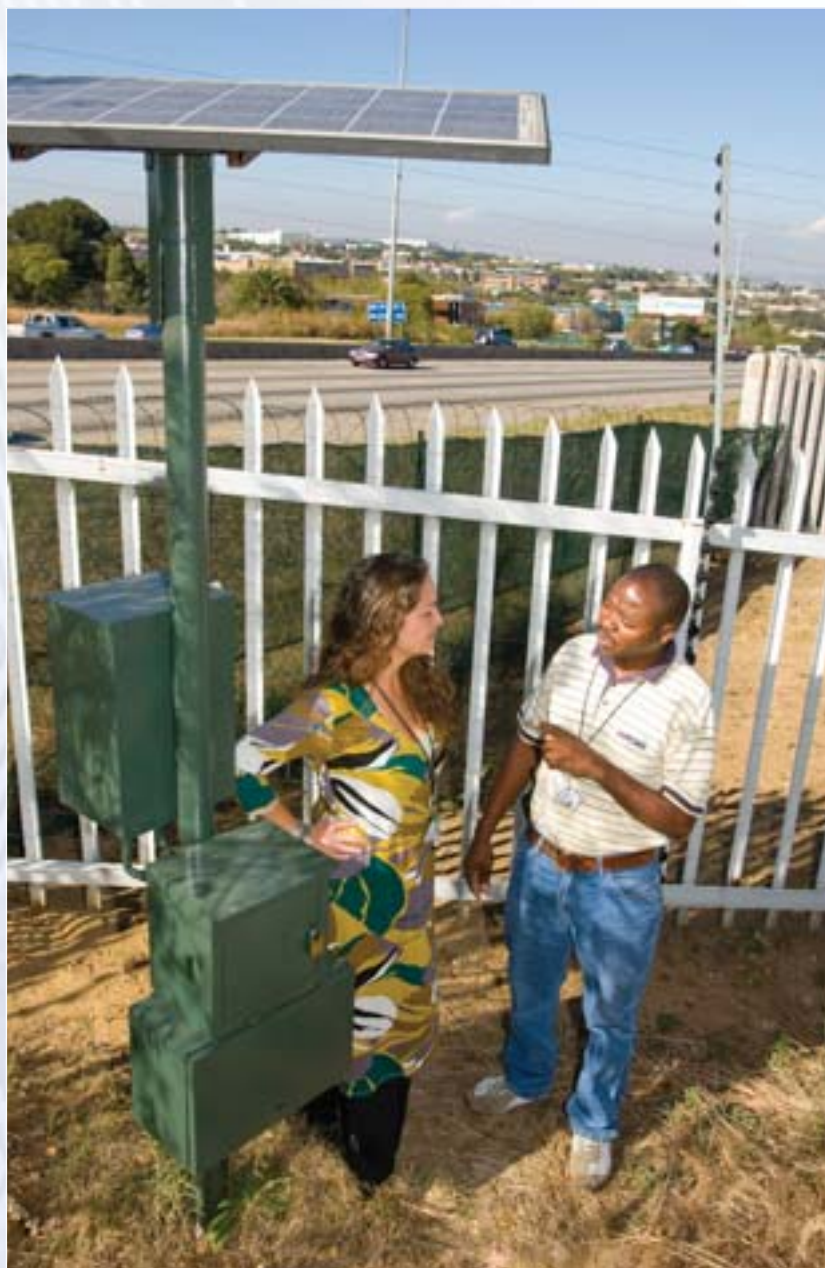
Ronel Eksteen, Bytes Business Park facilities manager and Kleinbooi Mashiyé, assistant, at the solar powered security fence at Bytes Business Park.
