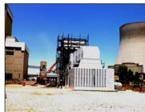
Above: One of two 20MVA OCGT Units at installed at Kendal
