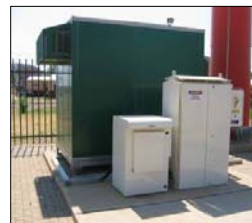
Above: 5kW Fuel Cell Systems
